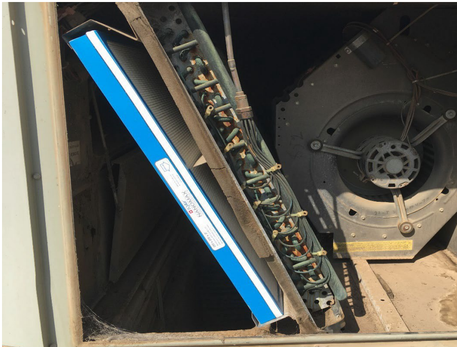
Caption: HVAC unit with IQAir High Performance Filter (Heber School, Heber, CA)
